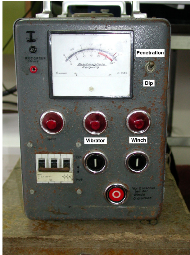
Fig. 17: Switch- and controlboard of the vibro-system. Determination of dip and penetration (top), as well as control of operation of vibrator and underwater winch (bottom).
